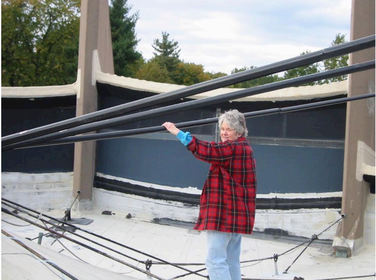
Cables covered with plastic slotted plastic pipe to prevent water flowing down inside the wire cable to the hub and then into the sanctuary. Janice Newton assistening 10/29/2005
