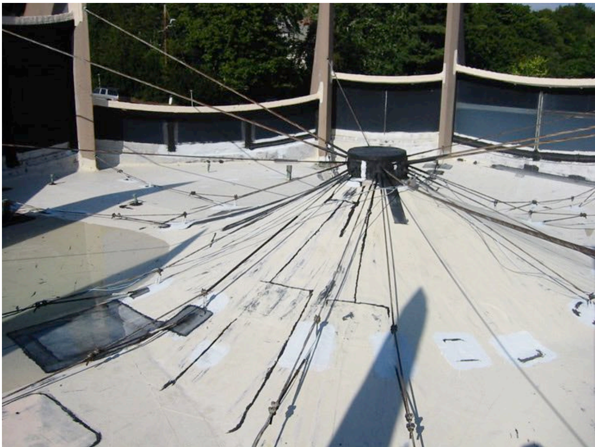
This is the roof. If you look carefully, you will see a lake on the left side! 2005
