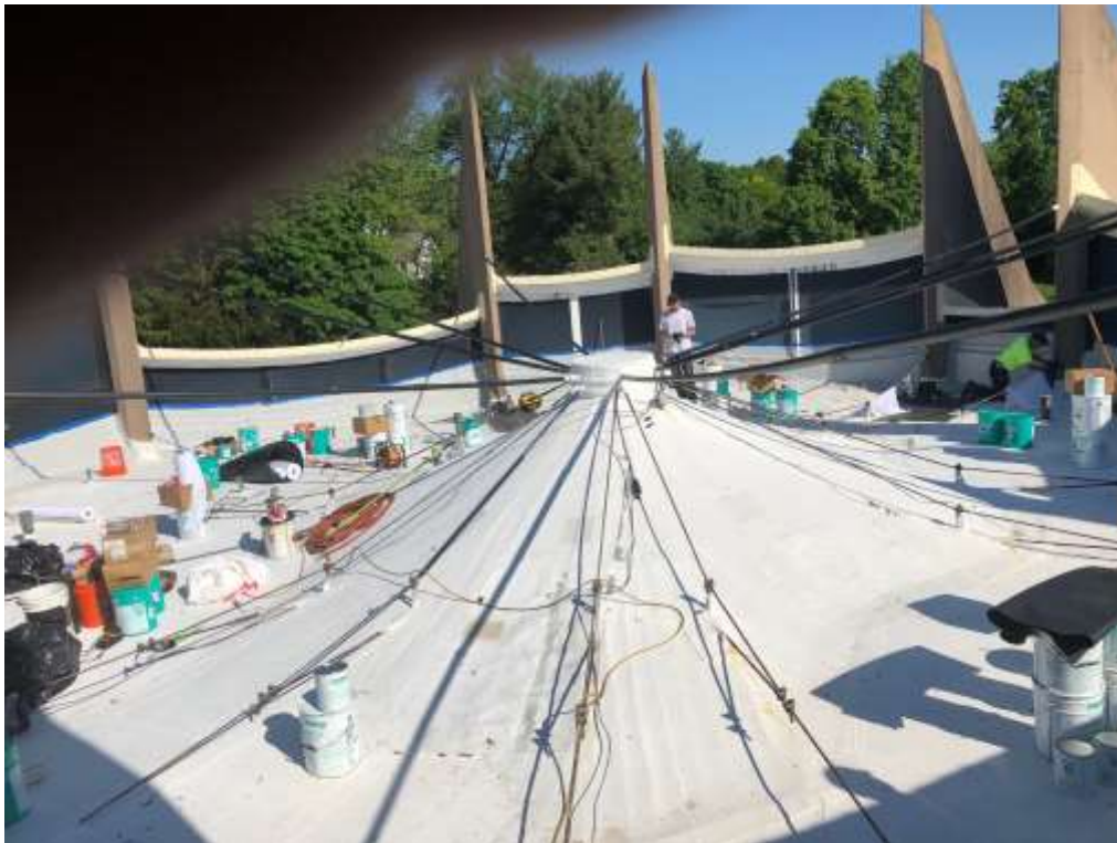
In 2018 a new methodology was employed to repair, recover and improve the roof. Here the contractor is surrounded by buckets of fluids and equipment used to apply a new tough membrane covering the entire roof (May 2018).
