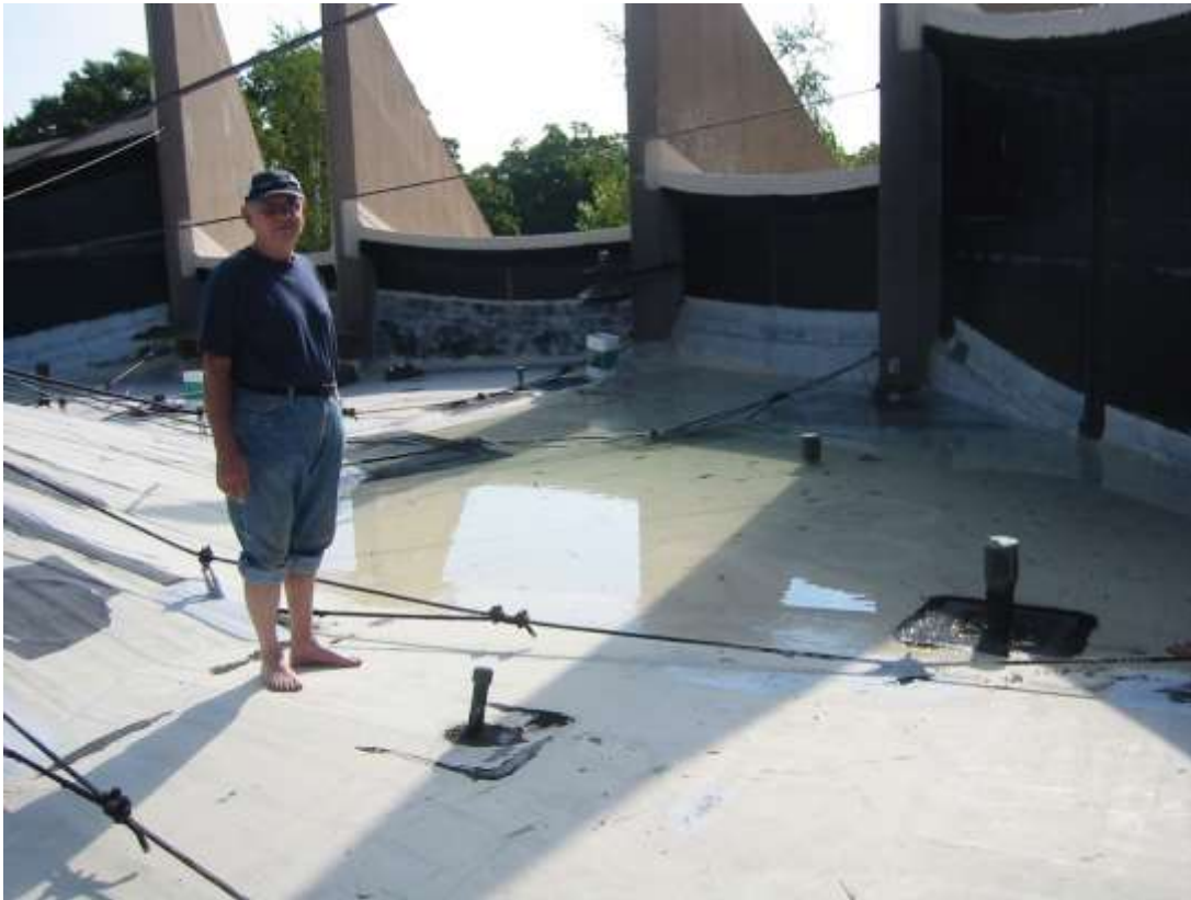
Ponding on the roof continued to be a problem because the drains needed to be improved and debris removal, freezing within, and such matters needed to be prevented. Here Stu prepares to enter the lake and open one of four drains. This particular drain was relined with hose to prevent the leak inside Servetus (October, 2005).
