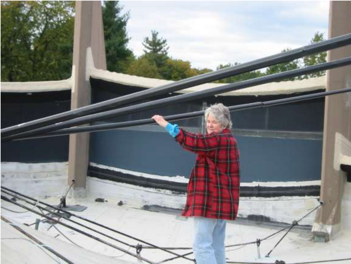
We discovered rain falling on the cables supporting the roof drained down into the support hub, and from there entered the Sanctuary, so we covered the cables in 2005, and that helped.
